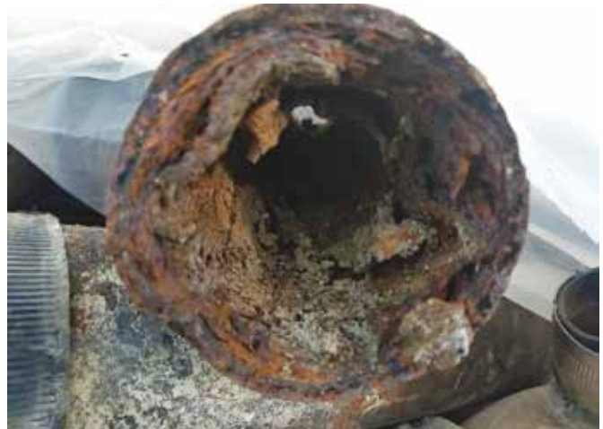
A 4-inch pipe loses capacity because of corrosion and debris.
