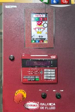
Painel de Controle
