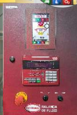
Painel de Controle
