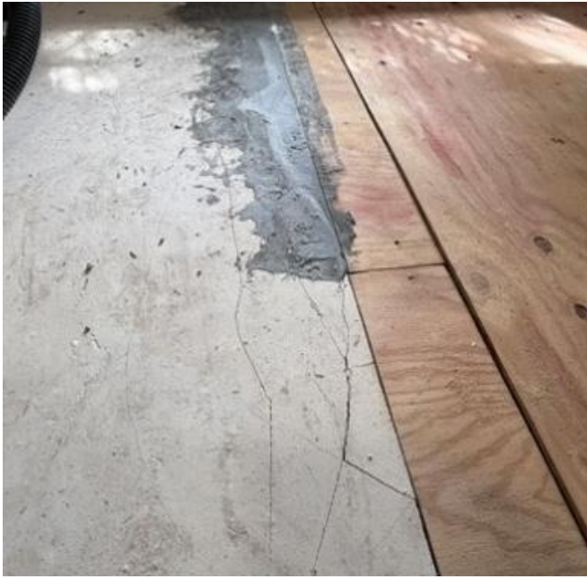
4. Unapproved wood plyboard
