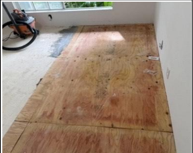
4. Unapproved wood plyboard
