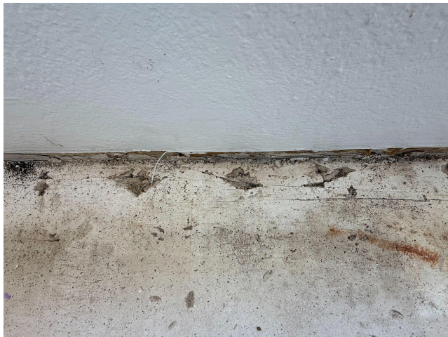
1. Damaged gypsum from carpet tack strips
