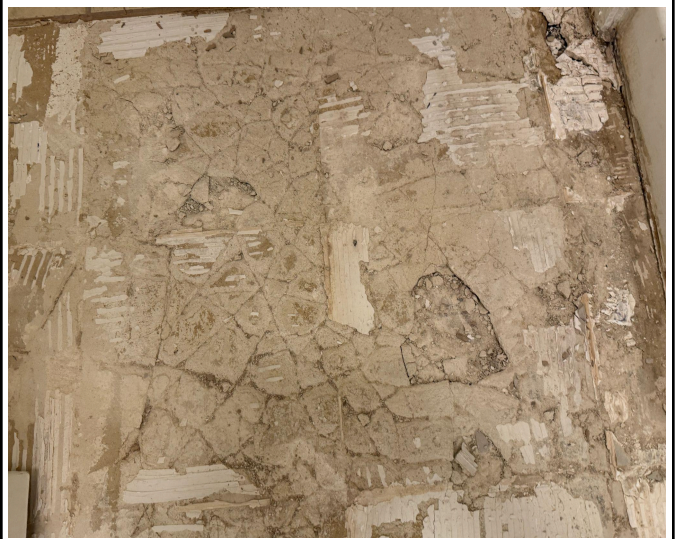
2. Main bathroom - gypsum damages
