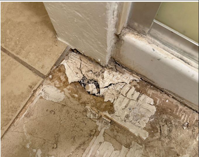
3. Main bathroom - gypsum damages, evidence of leaking shower door track
