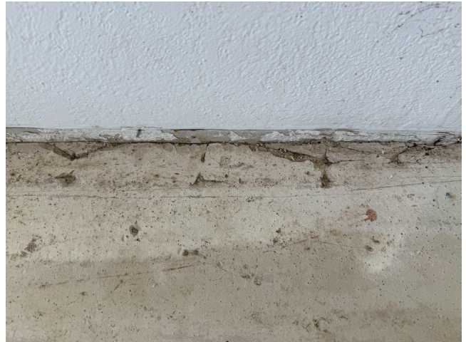
2. Damaged gypsum from carpet tack strips
