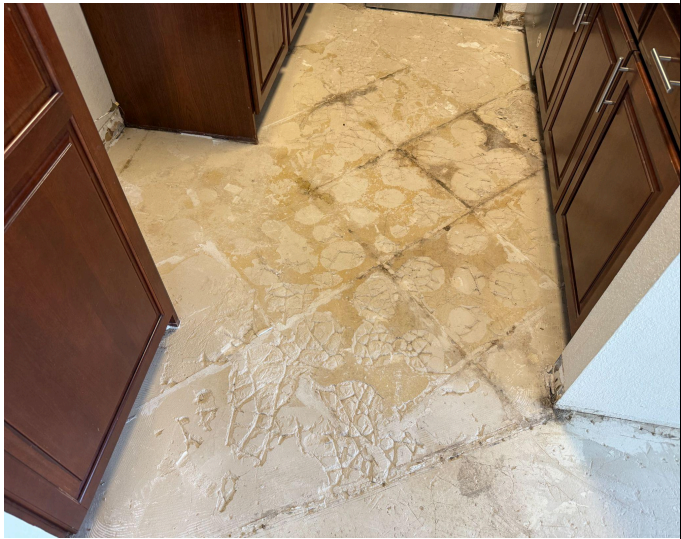
1. Kitchen - damaged gypsum.
