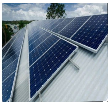
100kwp Solar ON-Grid System (3 Phase)
