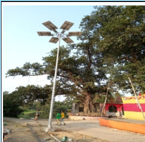
20watt High Mast Six Arms
