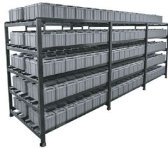
VRLA Battery Rack
