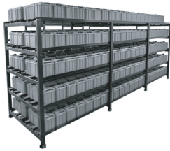
VRLA Battery Rack
