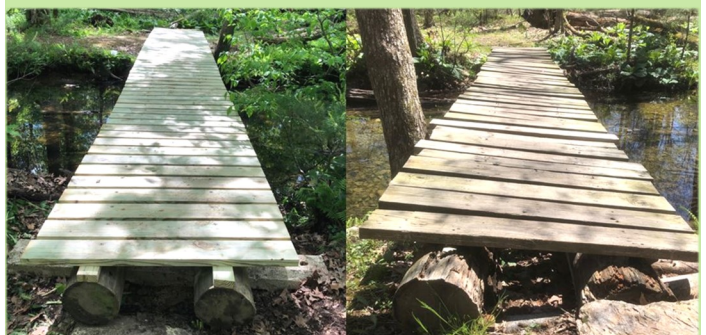
The just-completed trail bridge compared to the long-serving bridge that had been repaired many times in recent years!
