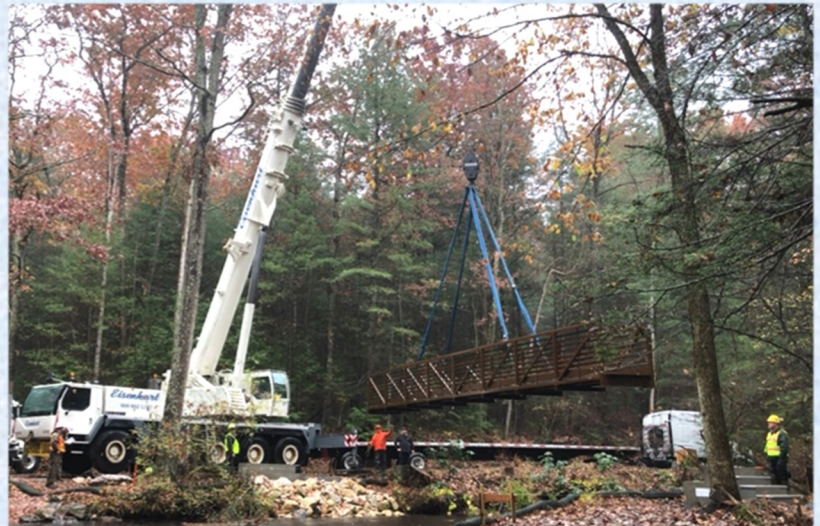
A 115-ton crane was used to position the bridge across Mountain Creek
