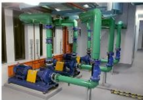
PUMP & MS PIPING
