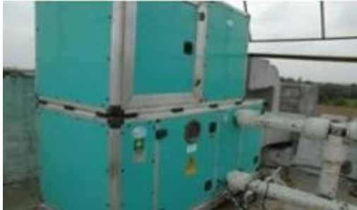
AIR HANDLING UNIT
