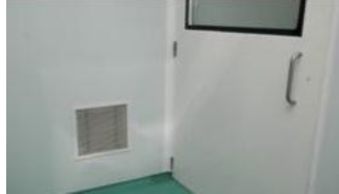
RISER FOR CLEANROOM/OT & DOORS
