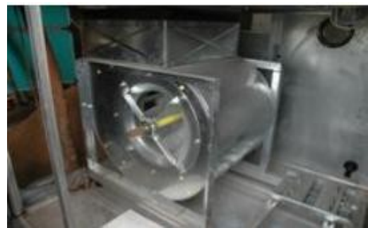
AHU FAN SECTION WITH DUCT FIXING
