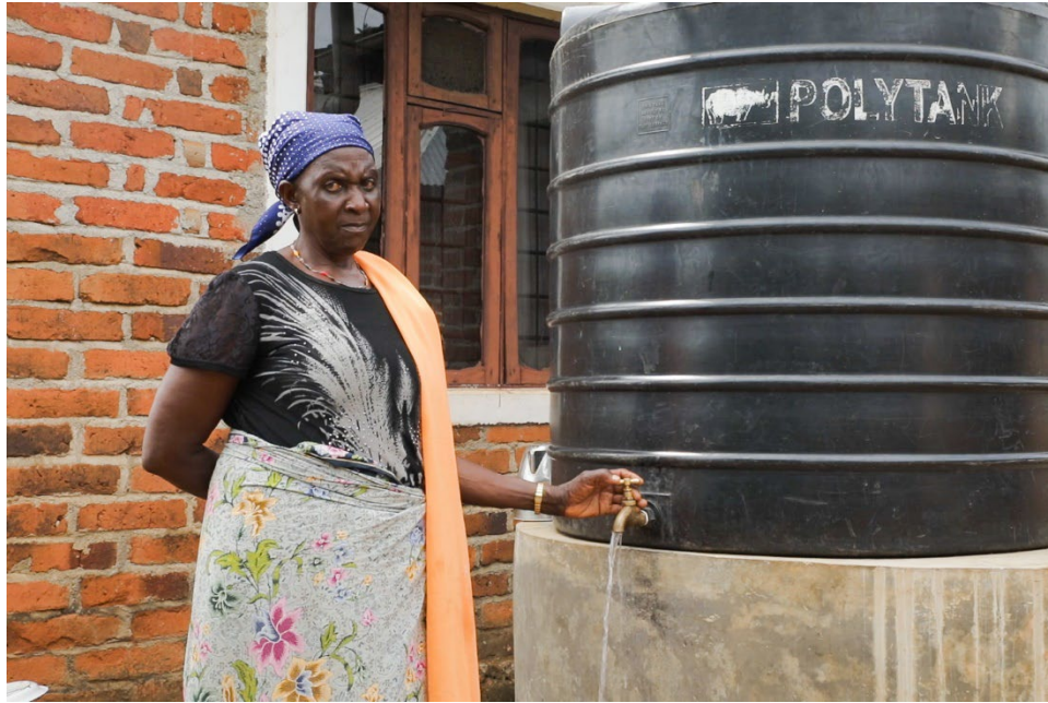
Pastor Tukupasia Bugali's domestic water harvesting tank
