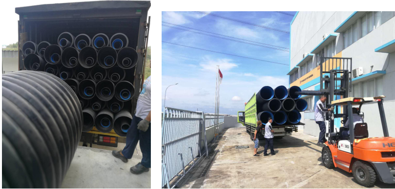
Yoyic factory(Cikarang) used shuanglin pipe as sewage system
