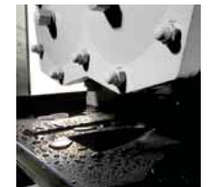
Gland water and drainage water is automatically caught and disposed by means of a bund.
