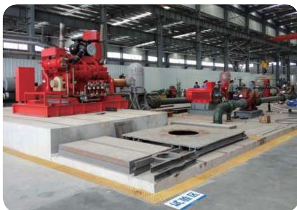
Pump and foam system testing station
