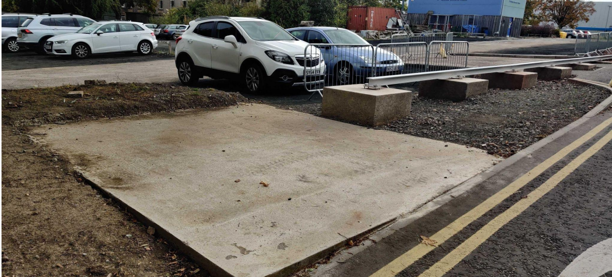
Figure 9.2: I-beam access point concrete patch.
