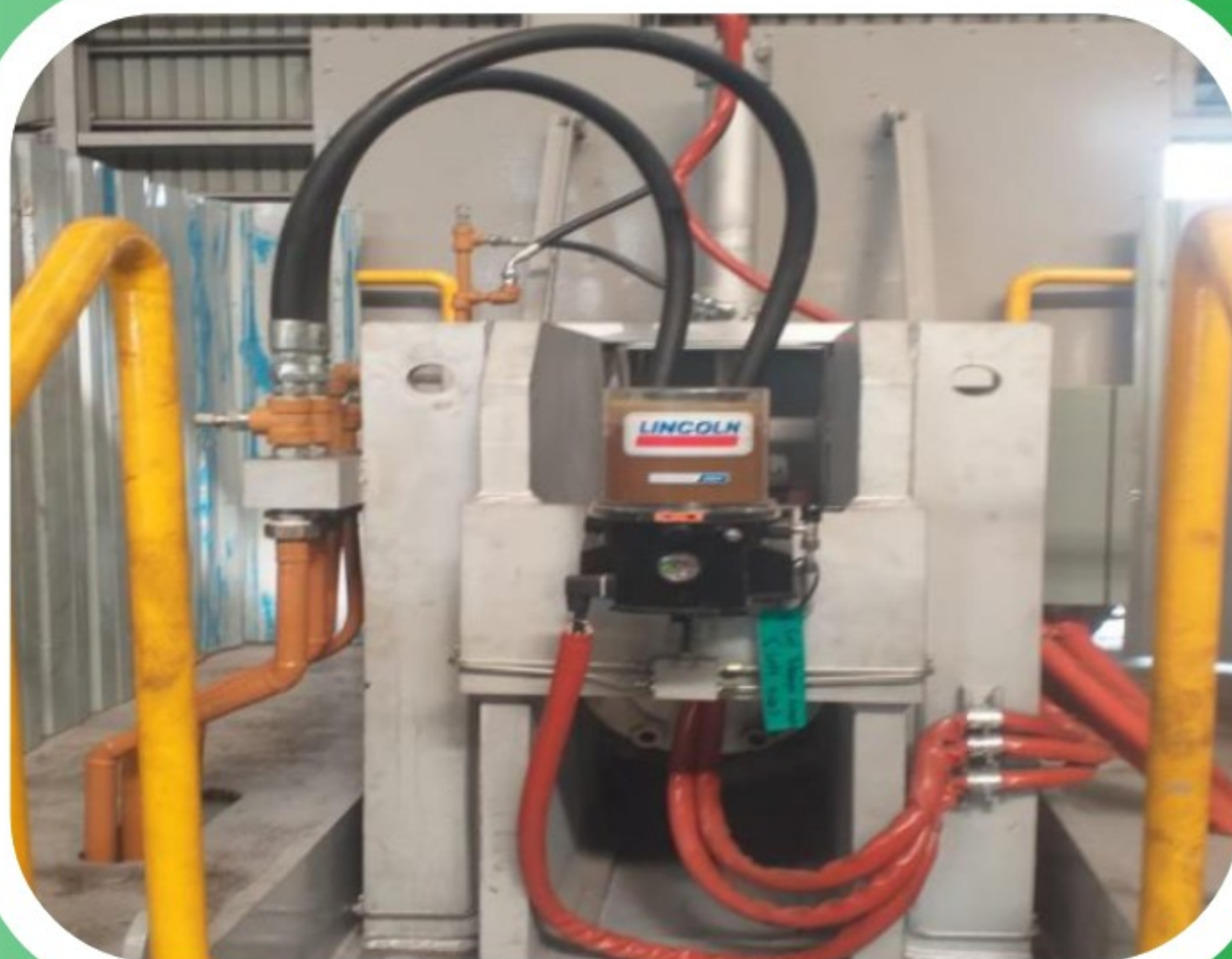
■ Koil Telescope Equipment PT. KRAKATAU POSCO
