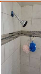
Location: 1ST FLOOR BATHROOM
