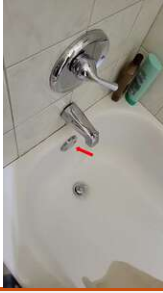
Location: 1ST FLOOR BATHROOM
