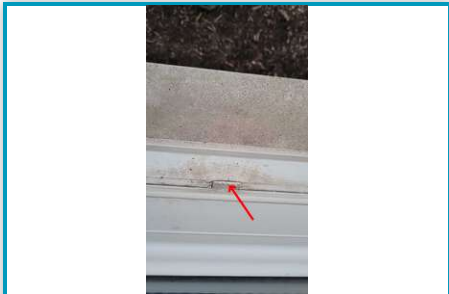
Location: LEFT SIDE FACING FRONT
