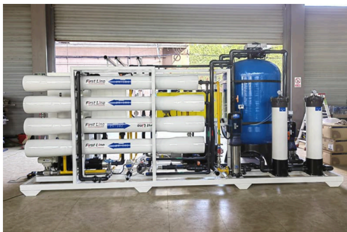
Packaged Sewage Treatment Plant
