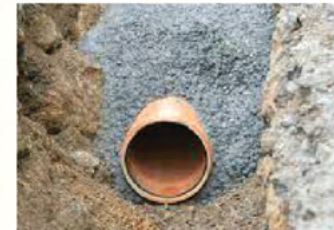
Underground sewer line
