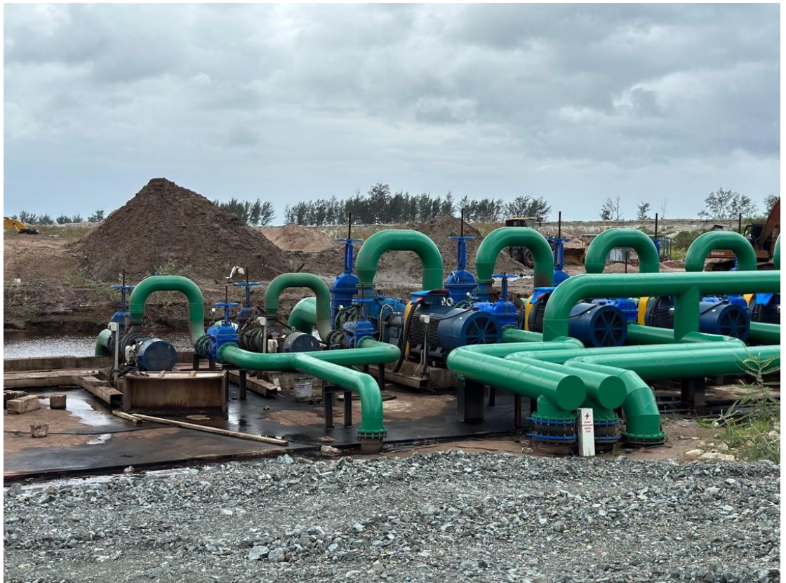
Photo 11: Use water or water that is received from the processing plant is gathered here at the Water Recycle centre (to be used in the Processing Plant)
