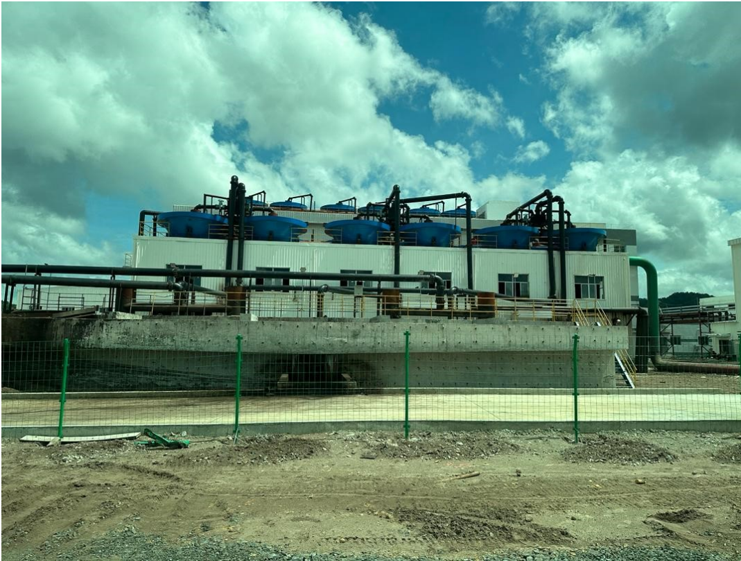
Photo 10: Silica Sand Processing Plant
