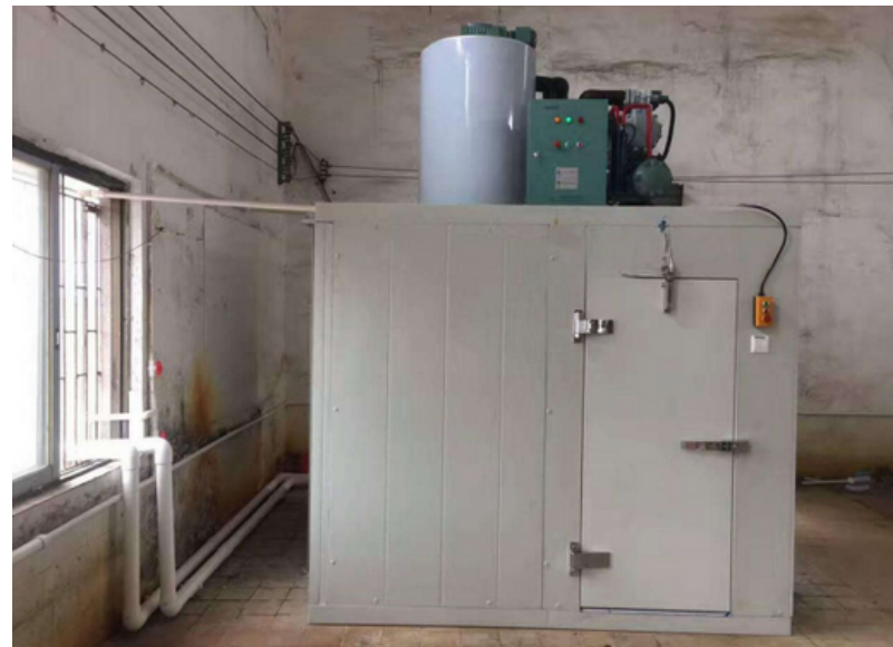
Ice Flake Machine application to Cold Storage
