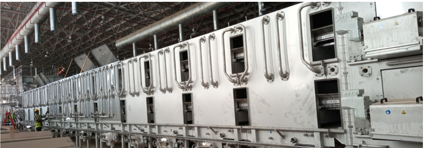
Installation of Pasteurizer
