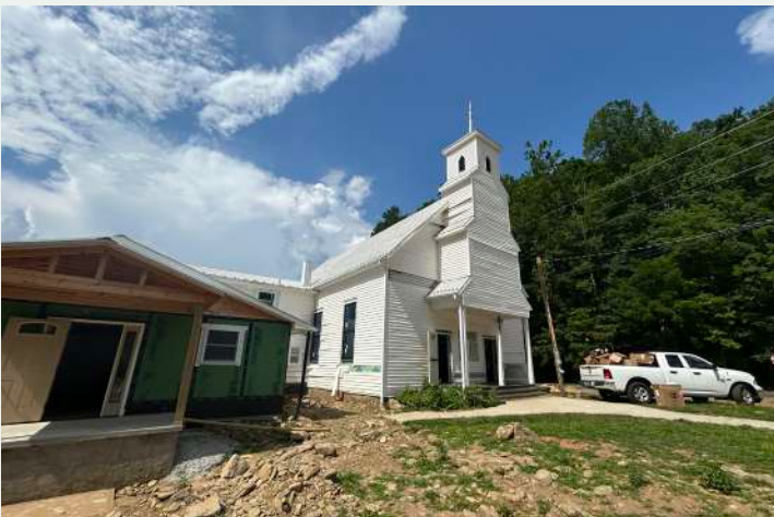
Figure 199. Oblique view of the south facade and west elevation of church, looking northeast from the front yard. Addition A covers the northern two bays of the church on this side.
