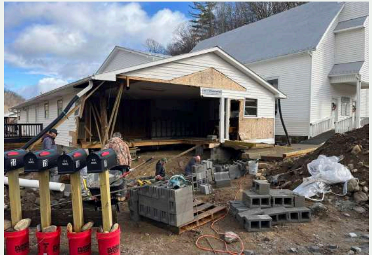
Figure 218. Hurricane Helene severely damaged the southwest corner of Addition B, requiring the Church to reconstruct a portion of its foundation, floor, and wall structure. (Laurel Branch Baptist Church, 2024(b))
