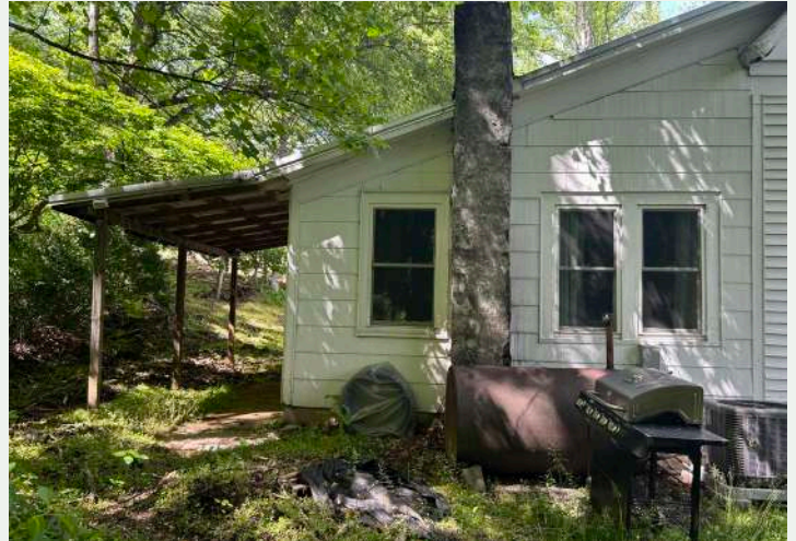
Figure 181. View of Addition C and covered patio on the south elevation, looking north from yard.
