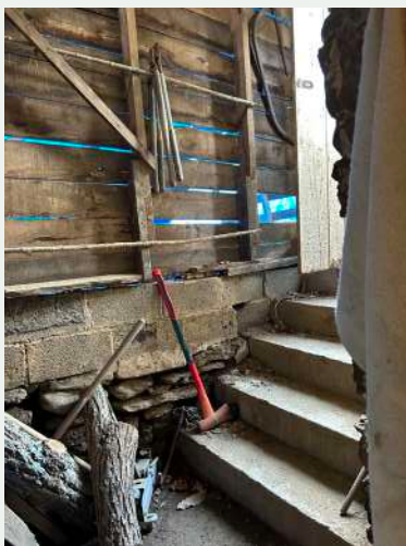
Figure 102. Enclosed exterior stairs of the addition, looking northwest from inside the basement.
