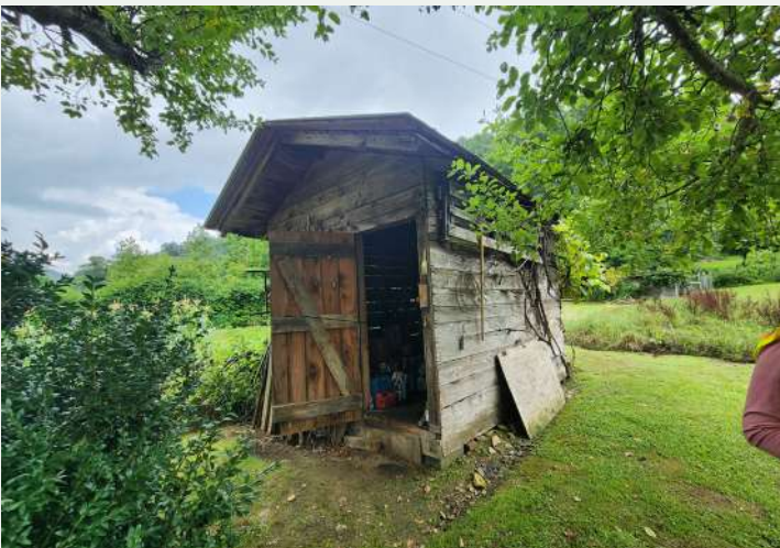
Figure 139. Smokehouse, now used as a garden shed, looking northeast from the backyard.
