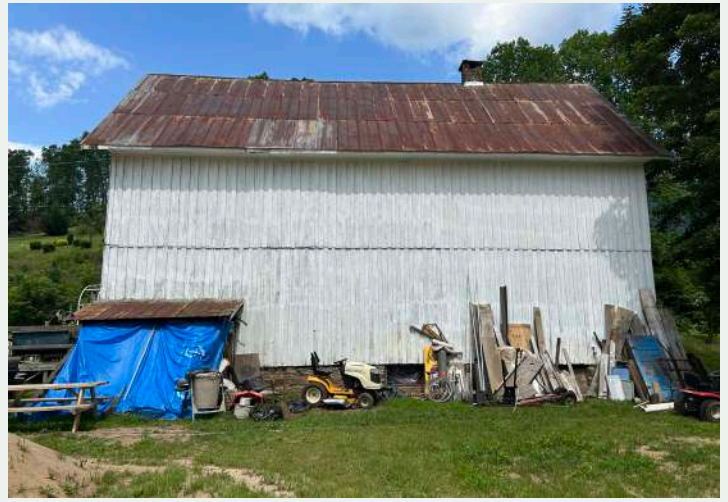
Figure 101. West elevation of the store, looking east from the yard. Note the lean-to shed addition covered by blue tarp at frame left.
