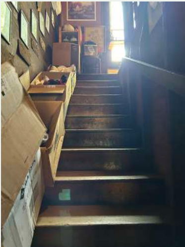
Figure 106. Historic wood stairs leading to the second level, looking south from the store.
