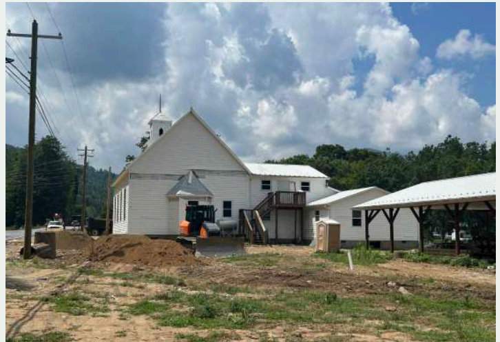
Figure 201. North elevation of the church and Additions A and C, looking southwest from the yard.
