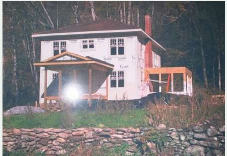
Figure 256. Reconstruction of the front porch and sunporch circa 2001. Note the new vinyl windows. (Boone 2025)
