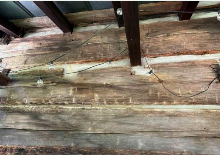
Figure 62. The historic logs show evidence of the reconstructed porch raising the height of the porch.
