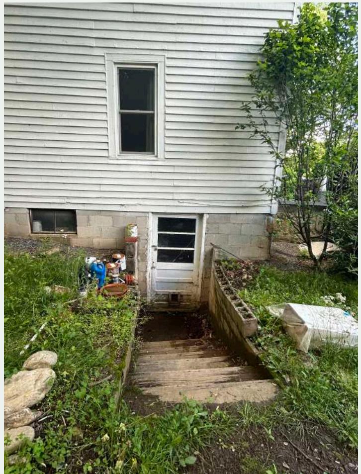
Figure 180. View of the basement entrance on the south elevation of the historic house, looking north from yard.
