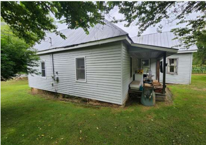
Figure 138. Oblique view of the south and east elevations of the house, looking northwest from yard.
