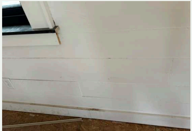
Figure 204. Shiplap covers the walls. Note the new casings and trim on the baseboard and surrounding the window.
