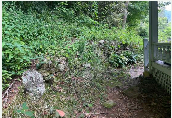
Figure 246. Stacked stone retaining walls behind the house, looking south from the backyard.
