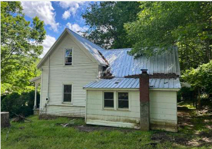
Figure 177. North elevation of the house, looking south from yard. The rear ell has been covered by Addition A, which projects to the north.
