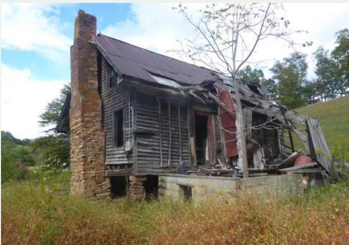
Figure 50. Oblique view of the west and south elevations of the tenant house, looking northeast from the pasture.
