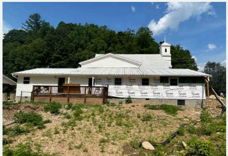
Figure 202. West elevation of Additions B (right) and C (left), looking east from the yard. The side gable of addition A extends above the ridge of Addition B.
