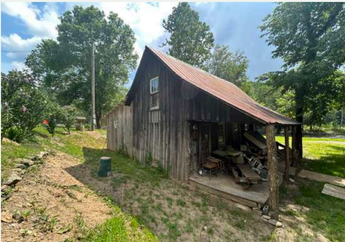
Figure 113. Oblique view of the east elevation and north façade of the tenant house, looking southeast from the yard.
