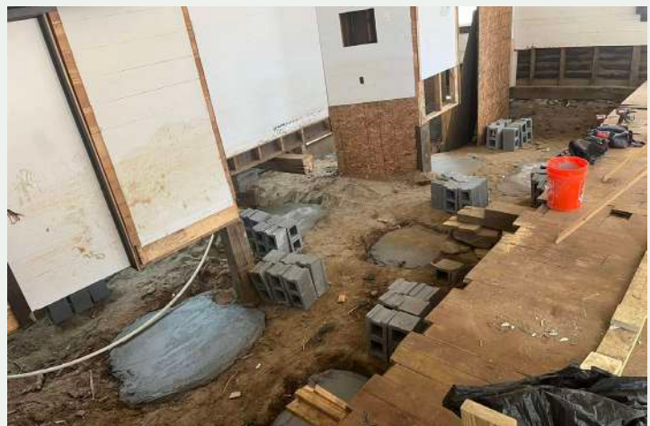
Figure 216. The historic wood floor had to be removed to pour new footings to support the altar. (Laurel Branch Baptist Church, 2025(a))
