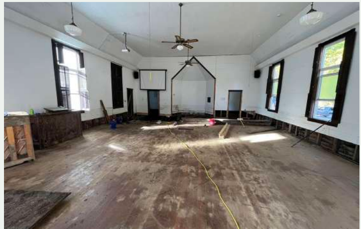
Figure 215. Interior of the church following Hurricane Helene. Note that shutters cover the historic window opening to the left of the side door accessing Addition A. (Laurel Branch Baptist Church, 2024)
