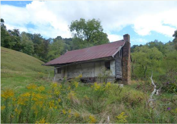
Figure 128. Oblique view of the north façade and west elevation of the Tenant House at the David Dellinger House (YC0028).
