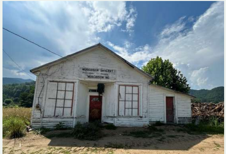
Figure 227. Southeast façade of the store, facing northeast from the front yard. Note the difference in the reveal of the weatherboard above and below the windows.
