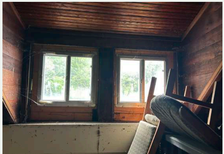
Figure 160. Shed dormer above staircase, looking east from the second floor central hall.
