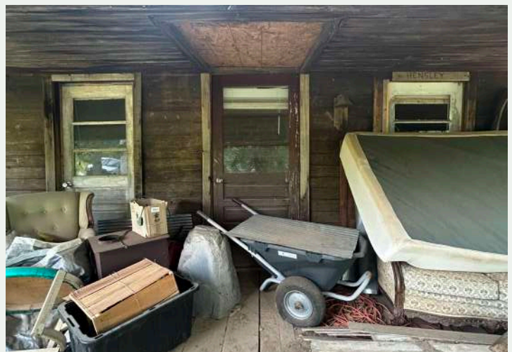
Figure 111. Three entrances across the tenant house's north facade. Note the plywood sheathing covering the opening above the central door.
