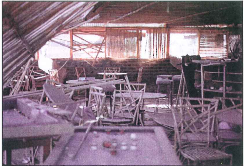
Stagecoach Inn after 122mm damage
