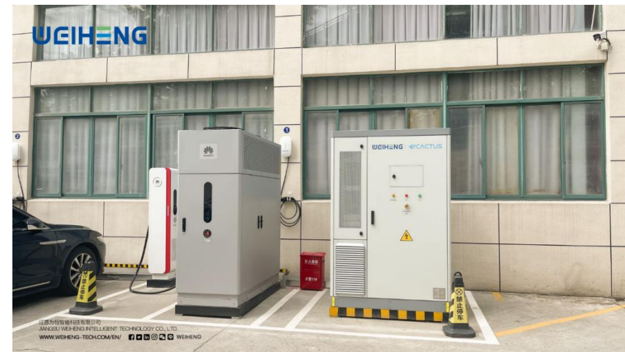
HUAWEI 600kW fast EV Charger case
