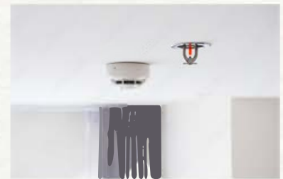
Sprinkler System & Smoke Detection System
