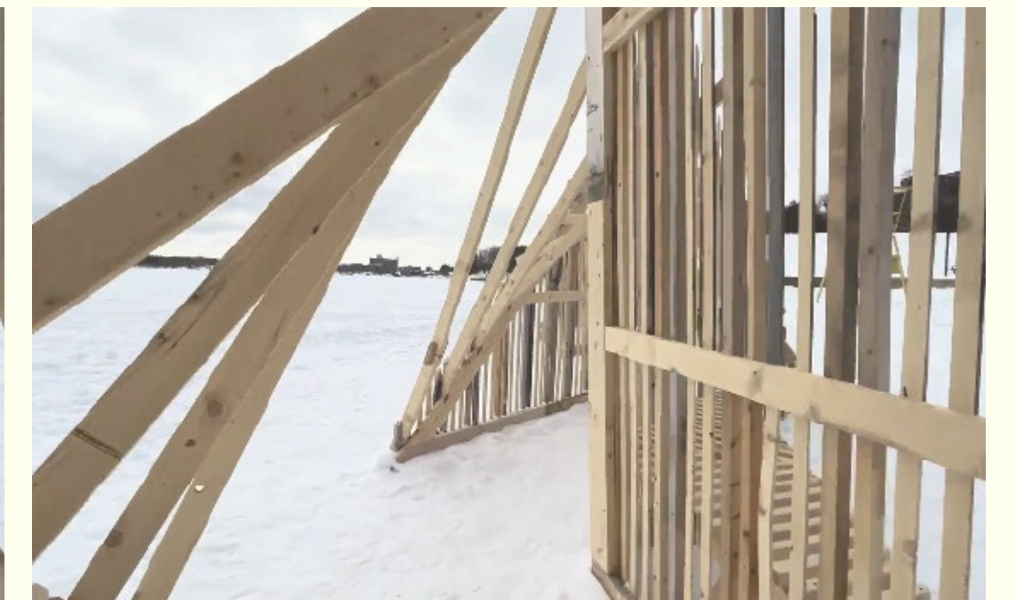
(Bottom) Interior Perspectives: Visitors must move with the rafters, enhancing the physical interaction of the experience. In addition, the gaps between each module can serve as entry points, but also help frame the surroundings.
