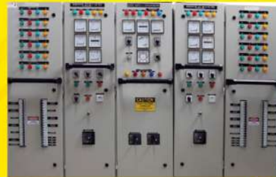
distribution panel (LVMDP)
