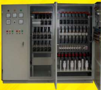
Panel Capacitor Bank
