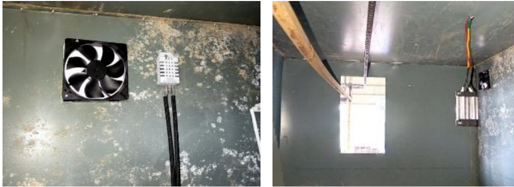
Figure 8. Internal View of the Drying Chamber
