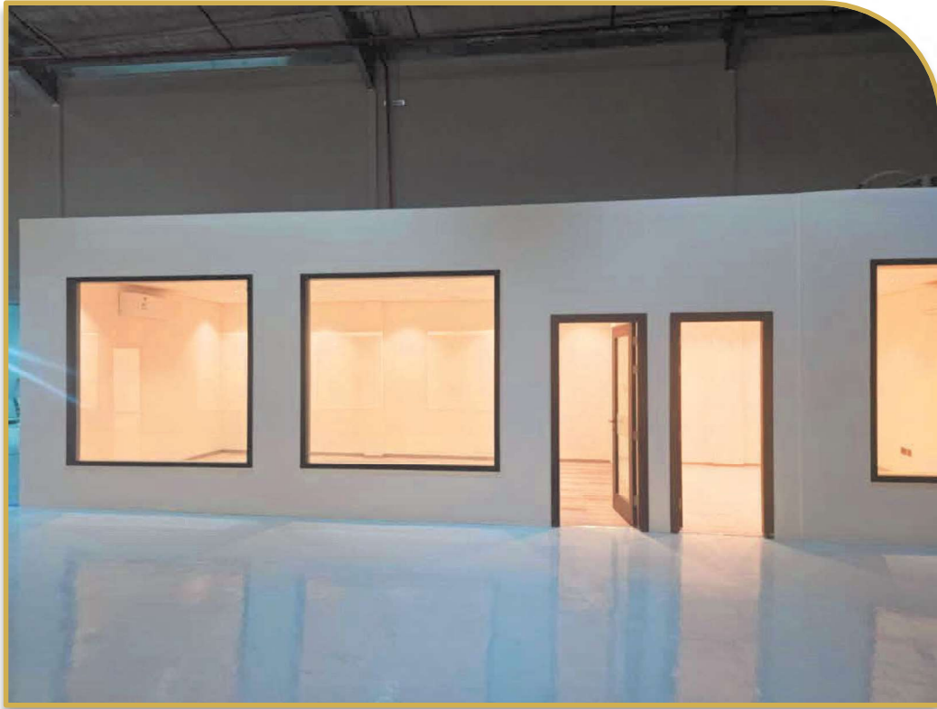
Factory Main Hall — Wide View with Sub-Rooms, Large Windows & Epoxy Resin Floor
