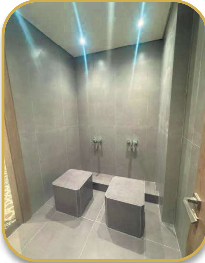
Ablution Room · Plumbing & Drainage
