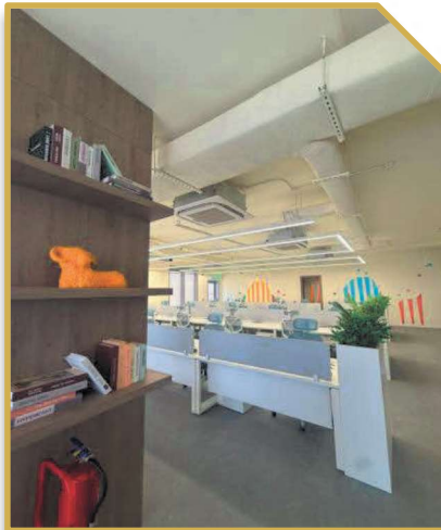
Open Floor View · HVAC Units
