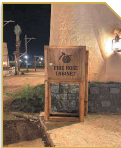
Fire Hose Cabinet · Heritage-Themed Casing Lantern
