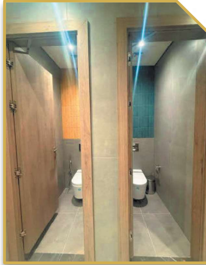
WC Cubicles · Full Sanitary Fit-out
