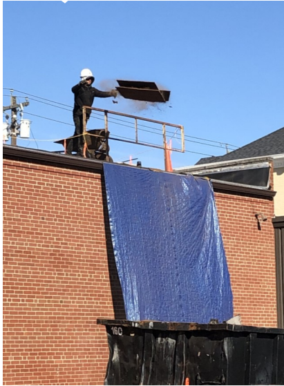
Thanks to the Friends of the Rose Garden Mission, major work was done to replace the roof
