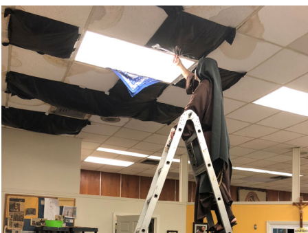
Sr. Clare covers up where the roof has leaked in to the Mission so we may control the "drip spots." Plans are in the works to replace the roof.
