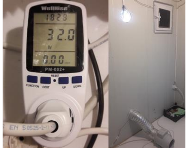
Figure 2. Position of the fans and air openings, and measurement of fan power with a wattmeter
