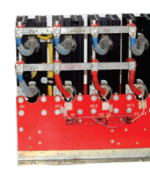
SCR EXCITER BRIDGE
