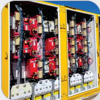
IGBT Control Panel
