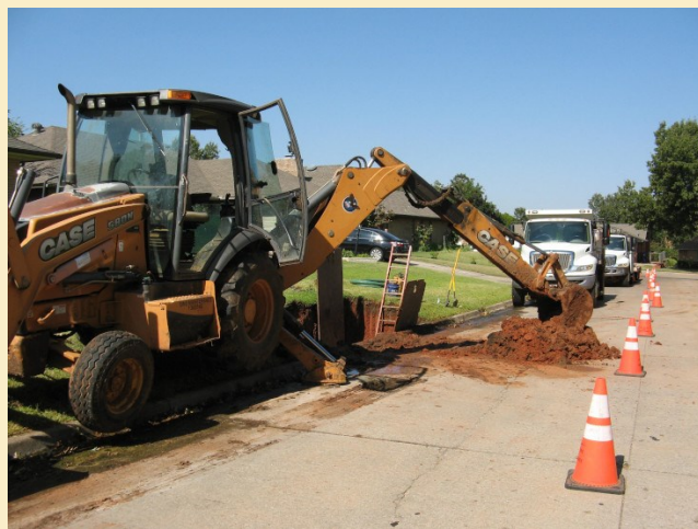
City utility workers arrived in our neighborhood in mid-September for some extensive work to repair broken water lines on N.W. 62nd Street and along a stretch of Tulsa Avenue. Our neighborhood is aging, and such leaks have grown more common in recent years as our water service infrastructure wears out. It's important to promptly report any water leaks you see as you drive or walk through the neighborhood. These leaks have potential to do great harm, and they do not go away on their own! You can call in the repair crews by phoning the city's Action Center at 405-297-2535 or emailing your report to action.center@okc.gov .
