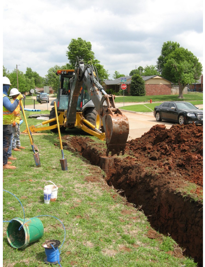
A crew digs a deep trench along Holiday Place in preparation for installing new water mains.
