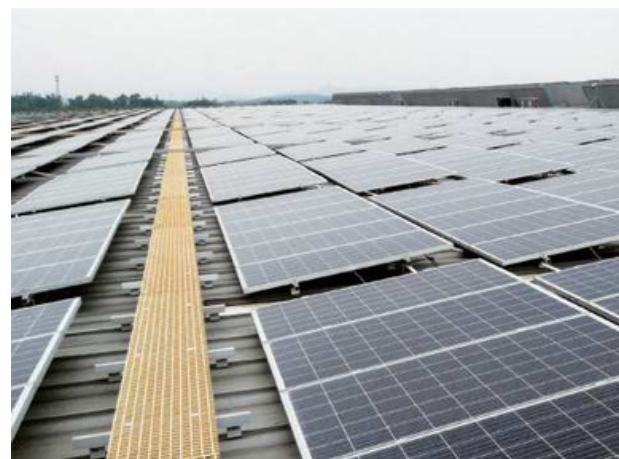
PV System Project Fukuoka, Japan | Year: 2021
