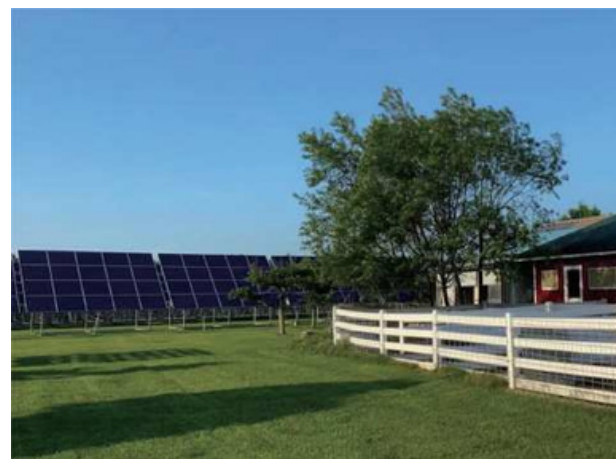
PV System Project Hokkaido, Japan | Year: 2022
