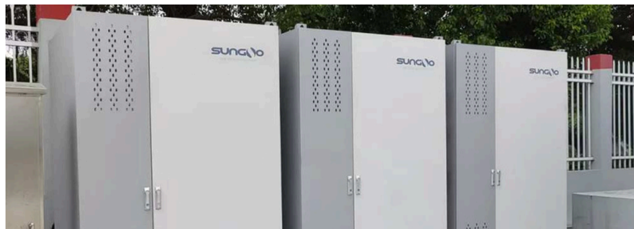
PV & Energy Storage System Project Wuxi, China | Year: 2023
