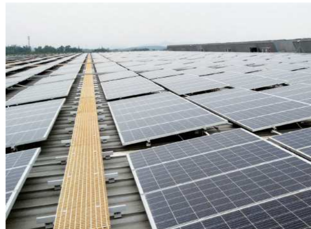
PV System Project Fukuoka, Japan | Year: 2021
