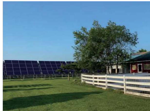
PV System Project Hokkaido, Japan | Year: 2022
