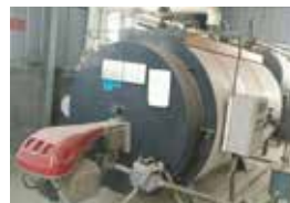
■ Air supply fan for boiler
