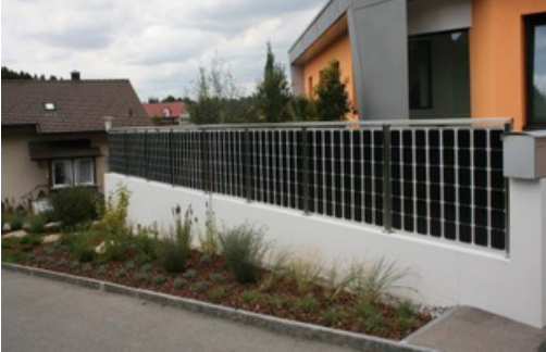
Integrated solar fence
