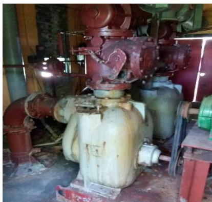
Sewer lift station needing rehabilitation
