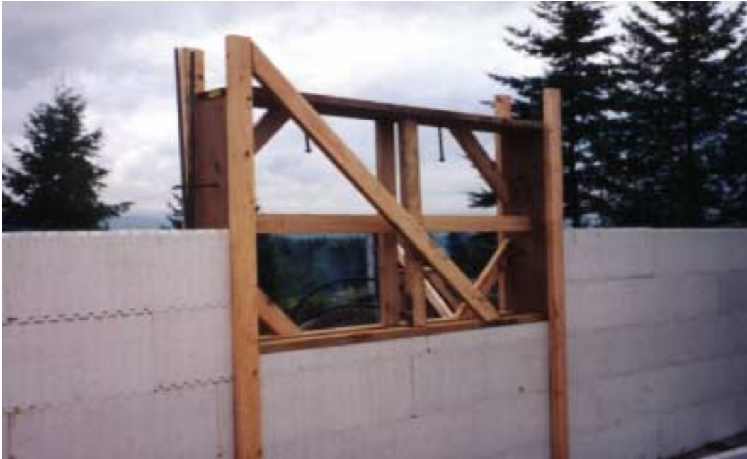
Doors and windows are set into bucks locked into the solid concrete.
