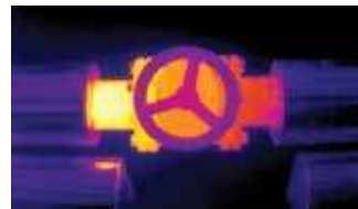
Thermal camera view of the uninsulated valve
