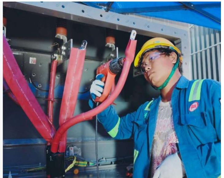
Electrician Cabel Panel / Lokasi 3100
