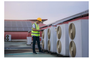
Heating and cooling
