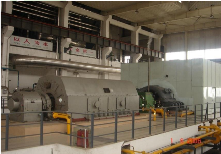
40 MW Steam Turbo Generator Set
