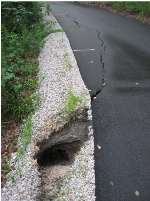
Sinkhole & road cracks from broken culvert near lot 6
