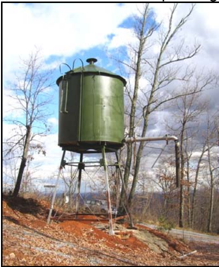
Water Tank installed near cell towers
