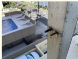
Construction Defect Investigation
